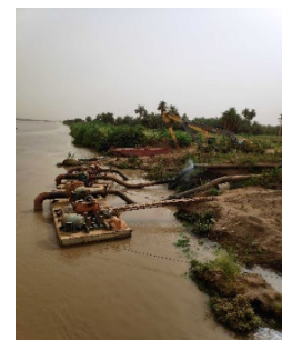
Taking water from the Nile using floating pump
